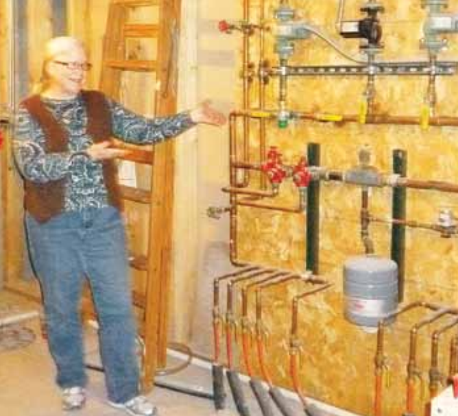
Phyllis Owan explains the challenge of sheet rocking through a maze of pipe and duct work in the furnace room that adjoins the child care space at Good Shepherd Lutheran church in Williston.
